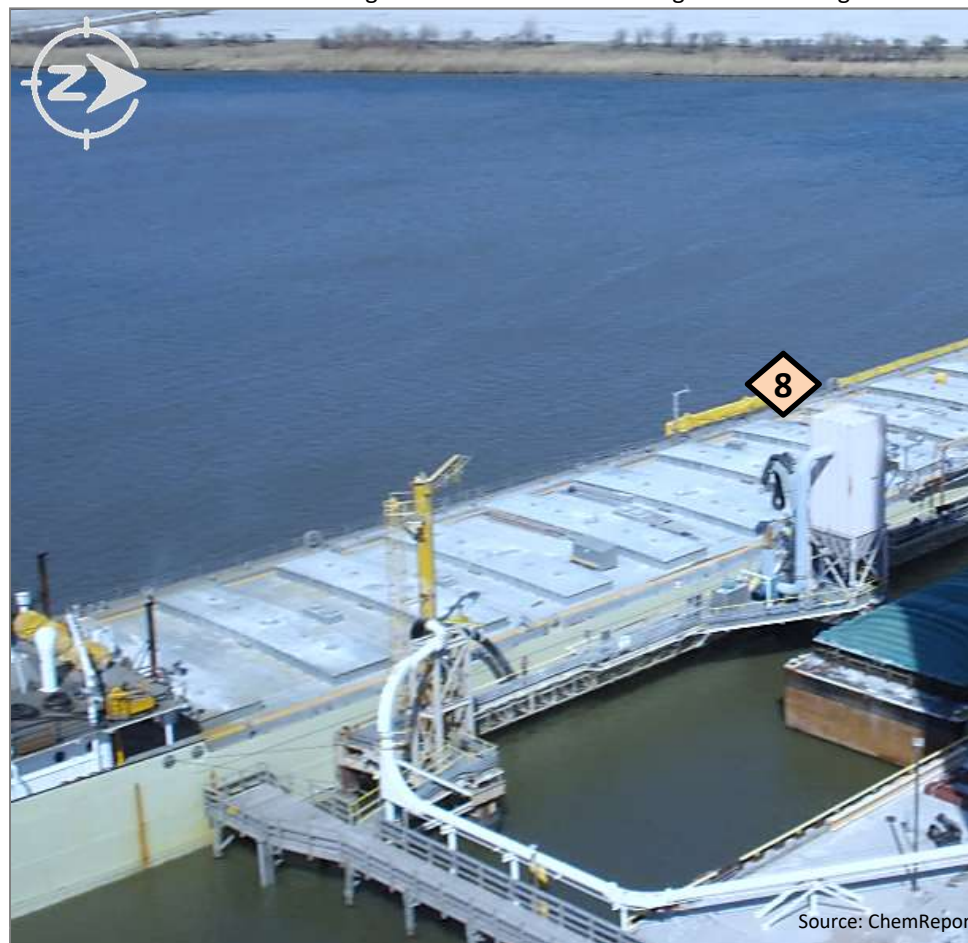
Showing Dust Collector No. 8 During Vessel Loading
